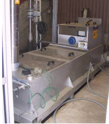
Figure 15 – Tank mounted Step screens
