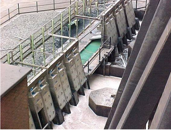
Figure 14 – SSV for cooling water intake
