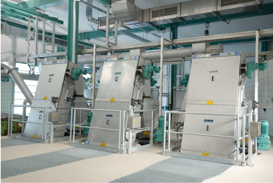
RakeMax® Multi-Rake Screens
