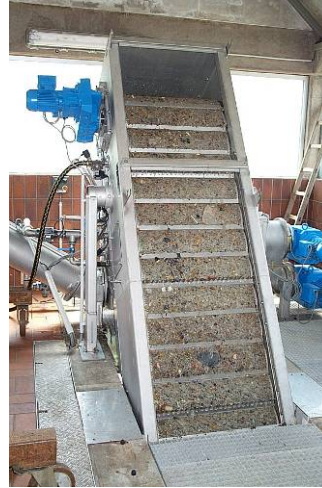
Figure 21 – Perforated band screen (covers removed)
