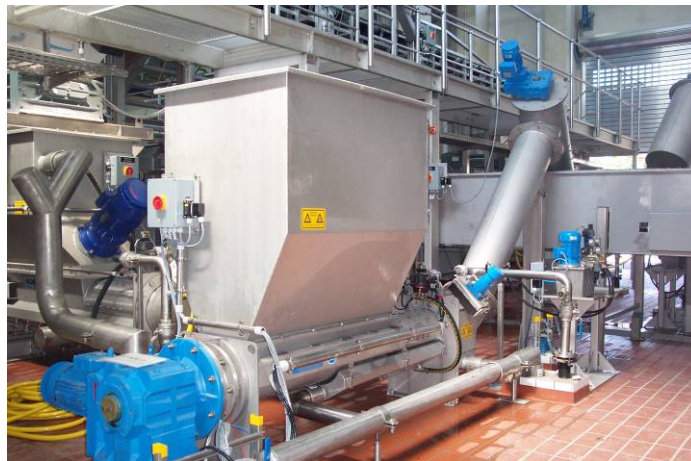
Figure 39 – Screenings washer/compactor with high pressure Compaction feature
