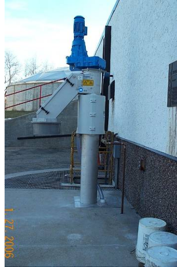
Figure 31 – RoK4 outdoor installation in Elroy, Wisconsin
